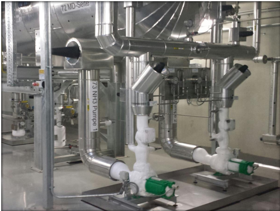
Installed Hermetic Refrigeration Pumps (image courtesy of Hermetic)
